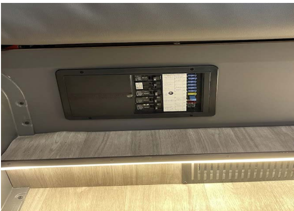
House 12-Volt Fuses (Located near the bed) -Typical View
