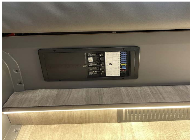
120-Volt Circuit Breakers -Typical View
